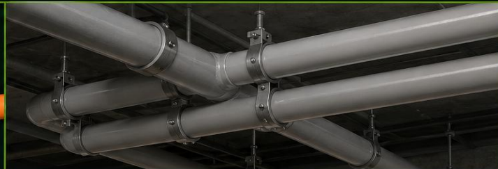
Double Containment Piping Above Server Rooms
