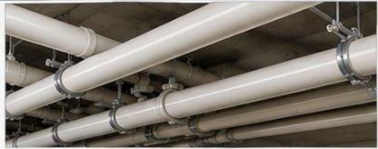
Chilled Water Piping
